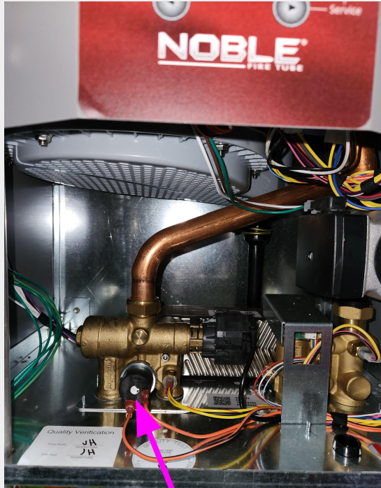
Pressure Sensor (near bottom left of boiler)
