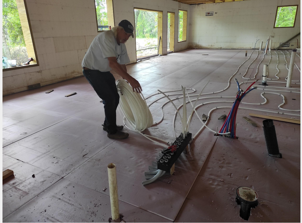
Pex Piping being rolled out on the pink foam on a new build.
