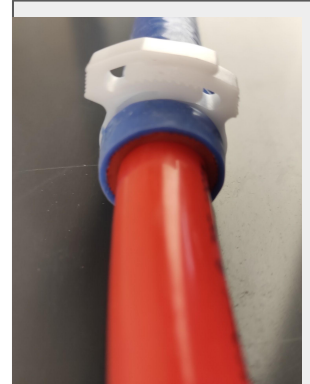
A securely connected blue tank hose to an orange pex pipe.
